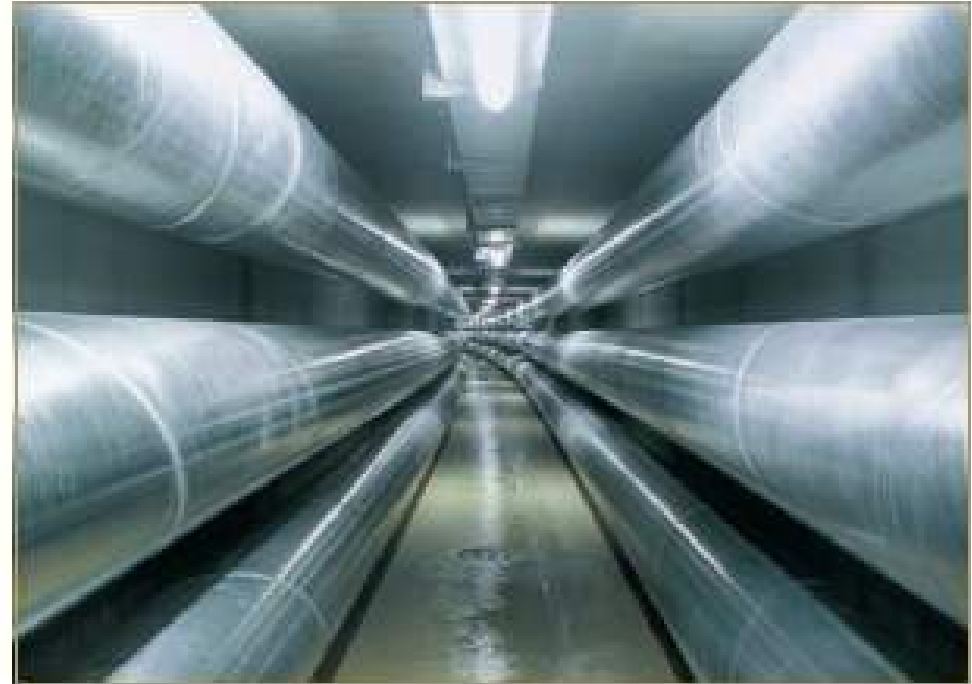
A gas insulated transmission line tunnel in Switzerland.
