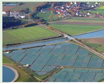
Central-Station PV: 6.3-MW Solarpark Mühlhausen (Credit: SunPower)
